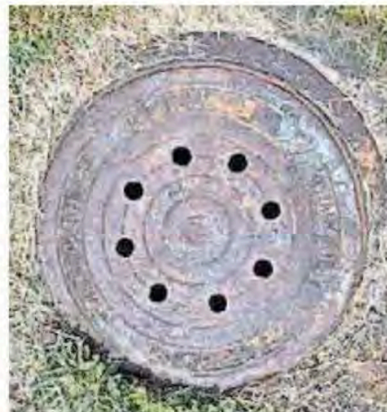
An aged manhole cover was installed before the Metropolitan Sewerage District of Buncombe County introduced newer covers with its logo design in 2010.
