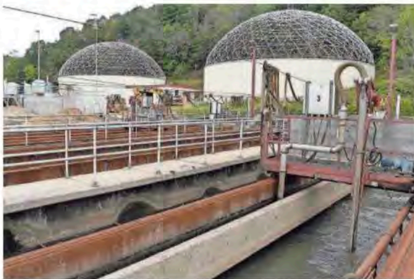
Wastewater is treated at the Metropolitan Sewerage District's water reclamation plant. ASHEVILLE CITIZEN TIMES FILE
