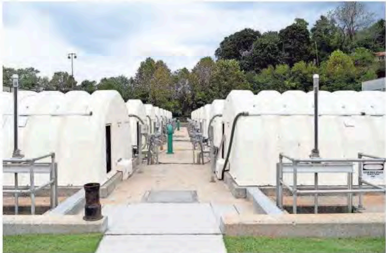
Rows of rotating biological contactors work as a step in the process of treating Asheville's wastewater at the water reclamation facility of the Metropolitan Sewerage District on Oct. 9, 2018. The facility has 152 rotating biological contactors. ANGELI WRIGHT/AWRIGHT@CITIZEN-TIMES.COM
