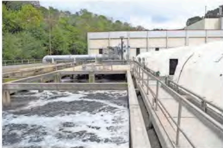
The Metropolitan Sewerage District of Buncombe County is participating in a statewide COVID-19 virus testing program. The treatment plant is in Woodfin. ANGELI WRIGHT/ASHEVILLE CITIZEN TIMES
