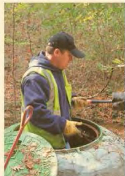
A worker with the Metropolitan Sewerage District of Buncombe County enters a raised manhole to inspect pipes. MSD cleans between 150 and 200 miles of sewer line annually with high pressure water jetting equipment.
