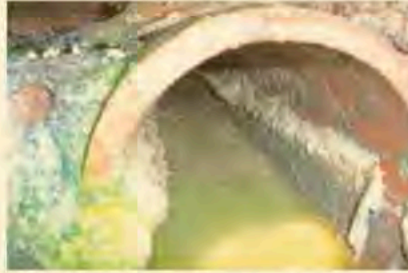
This photo shows congealed grease in an MSD pipe. PROVIDED BY METROPOLITAN SEWERAGE DISTRICT OF BUNCOMBE COUNTY
